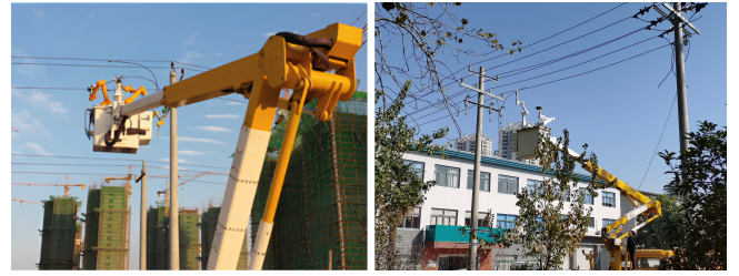
Figure 3. Aerial work robot for power grid tasks, equipped with two UR5 collaborative robot arms, lift into the air by bucket truck, developed by our lab.
